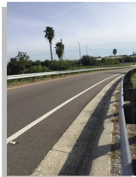
Figure 7: Pavement Condition Along EB Exit to 22nd St
